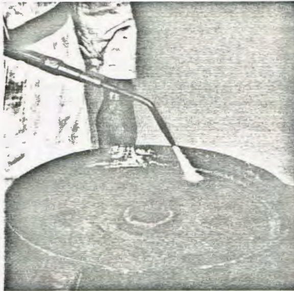
Step 3. Preheat casting in the heavy center portion of the bolster to prevent cracking.
