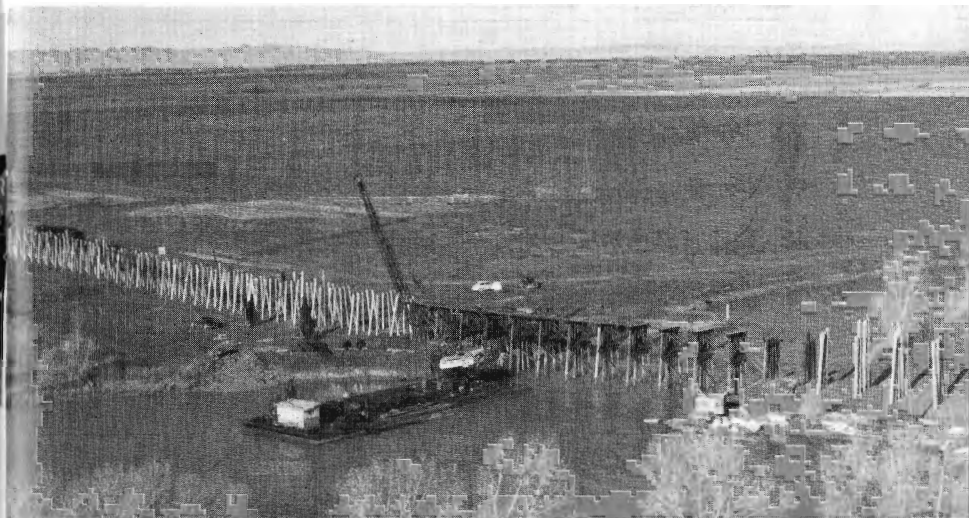
Some of the construction equipment was brought by barge to rebuild this section of the new trestle.
