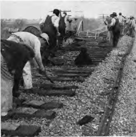
Power adzing and creosoting machines quickly prepare the ties for proper seating of new tie plates.
