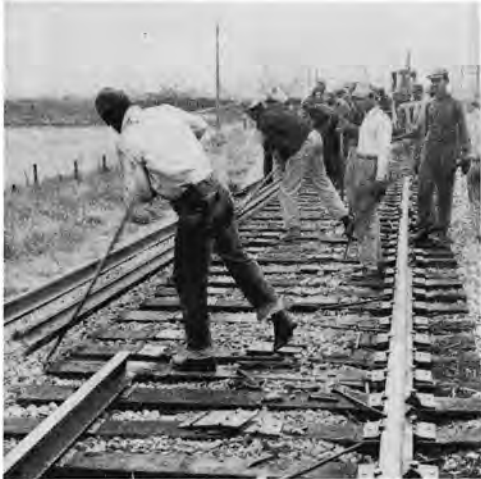
Barring out old rail after removal of the spikes is still more easily done by hand using crow bars.
