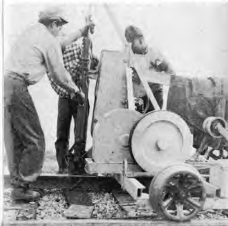
The removal of spikes is no problem for a modern power spike pulling machine, here shown in action.
