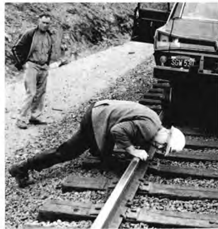
Below: The track seemed rough when the Hy-Rail auto passed this curve so Maury checks track alignment between Tunnels 5 and 6 and will report condition to roadmaster.
