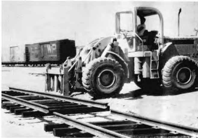
PRECEDING DOUBLE PAGE: A new Mannix ballast cleaner in operation east of Wendover and now working west of Gerlach.
