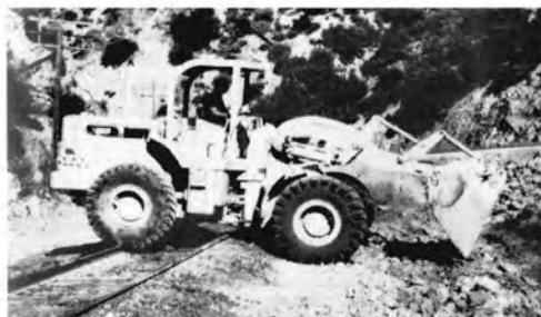
Below: Caterpillar 966B with front-end loader working in the Feather River Canyon.
