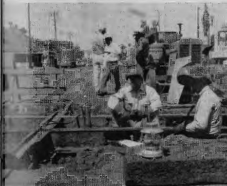
Welders Leonard Holt and C. W. Wilkins, with hoods, stopped long enough from making track repairs at Weber Avenue and Union Street for this photo by Lineman Brooks. In rear are Helpers J. T. Chavez, R. S. Gonzales, and (back to camera) Section Foreman R. Warren.
