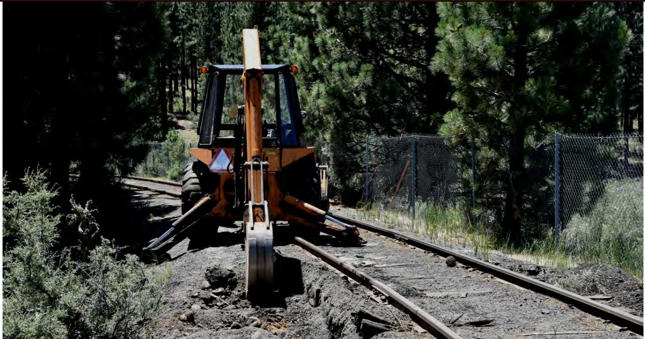
Don Nelson had stepped down for some lunch when Greg took this picture, it shows the work Don had done, but unfortunately not Don running the backhoe. Don did trenching the full length of the work site in preparation for tie replacement. A job well done and it will speed things up considerably. —Greg Elems Photo (30 June 2017)
