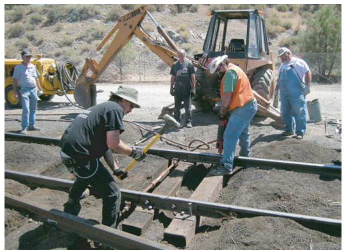
Kevin Caldwell and Eugene Vicknair square off with their chosen spike driving tools during the switch work. - Wayne Monger photo
