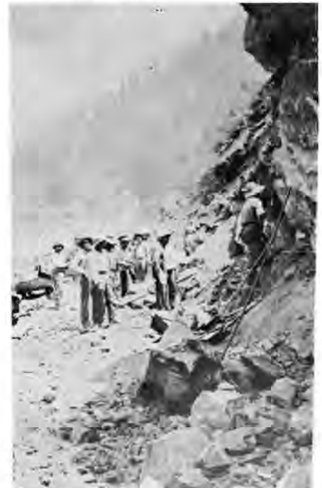
WP construction crews remove loose boulders on the walls of the Feather River Canyon during blasting in 1908. They were tough men, too, mostly lumber jacks and hard rock miners.
