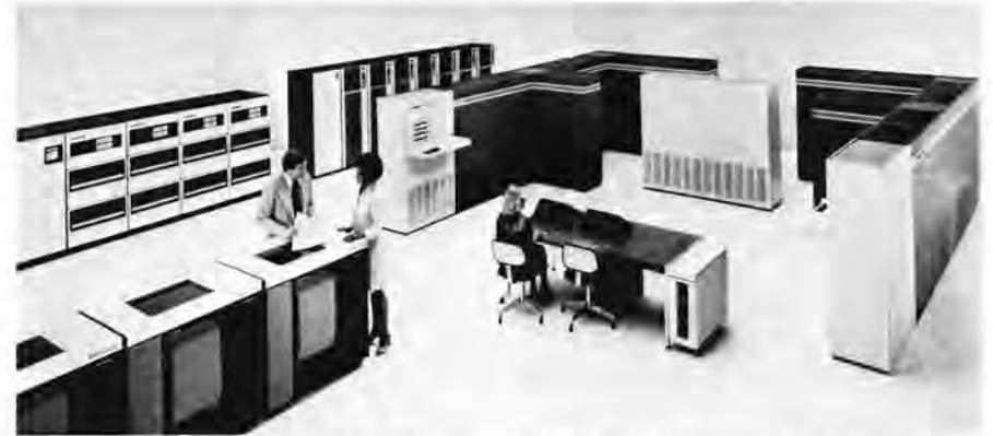
A view of WP's new Burroughs Computer System (B6817) showing (left back) disk storage units and tape drives and (left front) printers and control processors, and central control console; located at WP's computer center in San Francisco.
