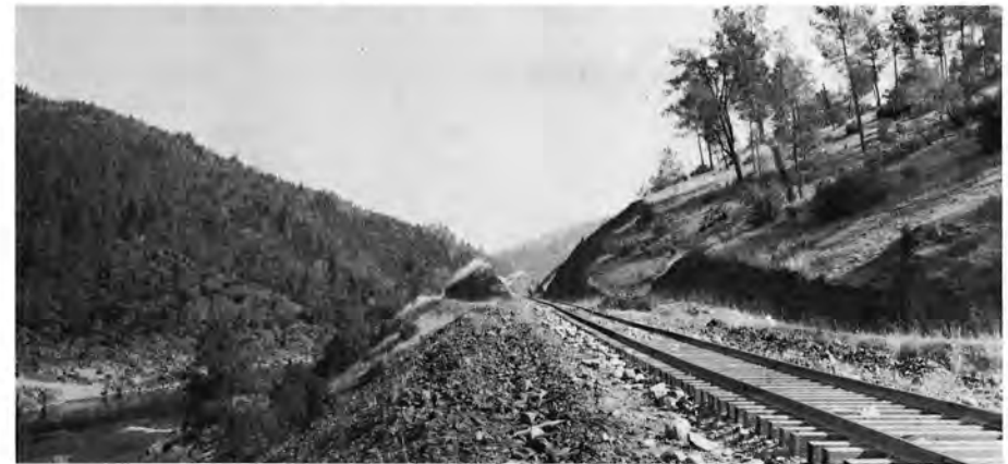
Early scene in the Feather River Canyon during the construction of the WP main line.
