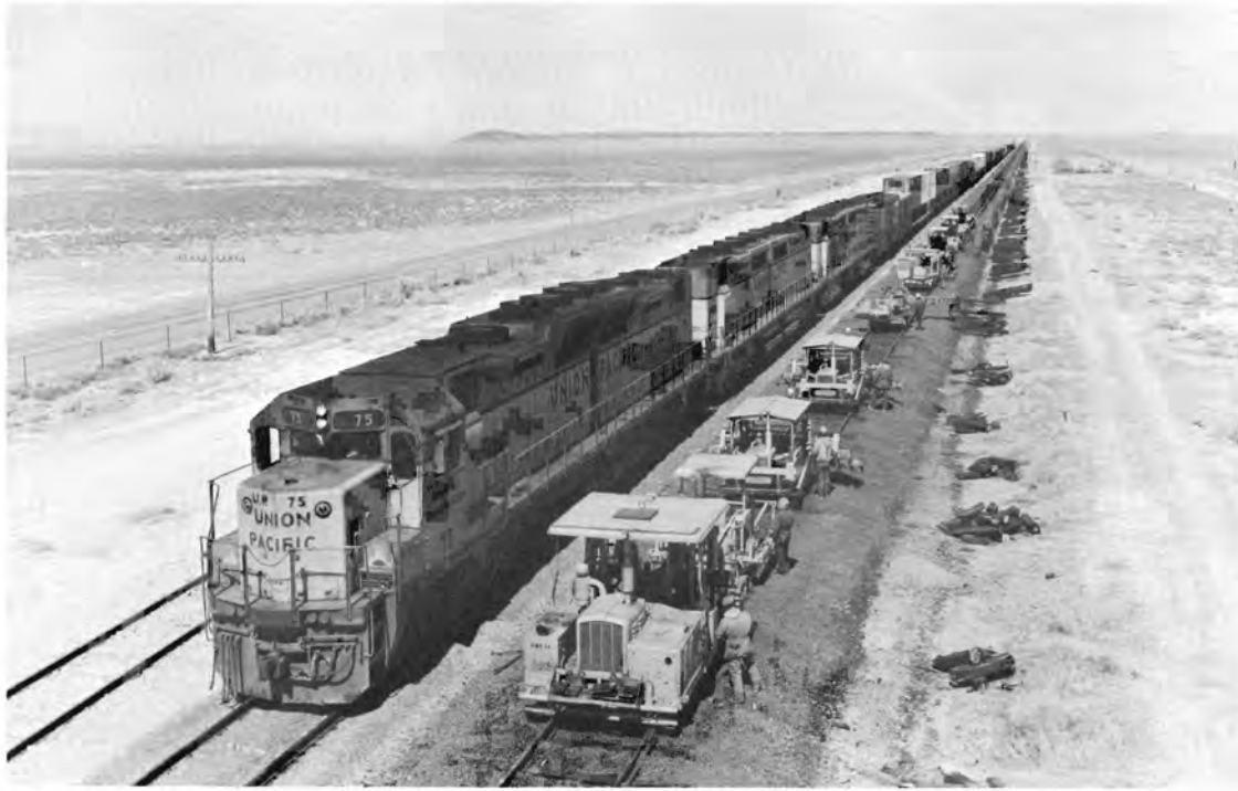
A Union Pacific freight train passes a track gang working near Neals, Utah. During 1979, UP spent $247.5 million maintaining its 9,700 mile rail system.
