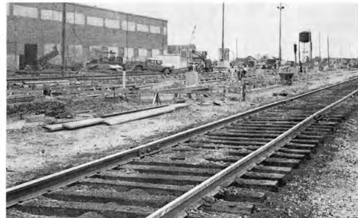
Area between new building and present "C" lead track in foreground (looking railroad west) will be occupied by engine servicing facility.
