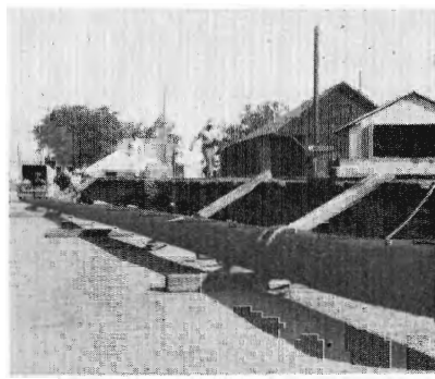
Tidewater Southern B&B gang N. S. Westfall, J. W. Alexander, J. J. Gonzales and R. B. Dixon (not in picture) just completed unloading a 110-foot radio antenna pole from two 60-foot flat cars at Modesto.
