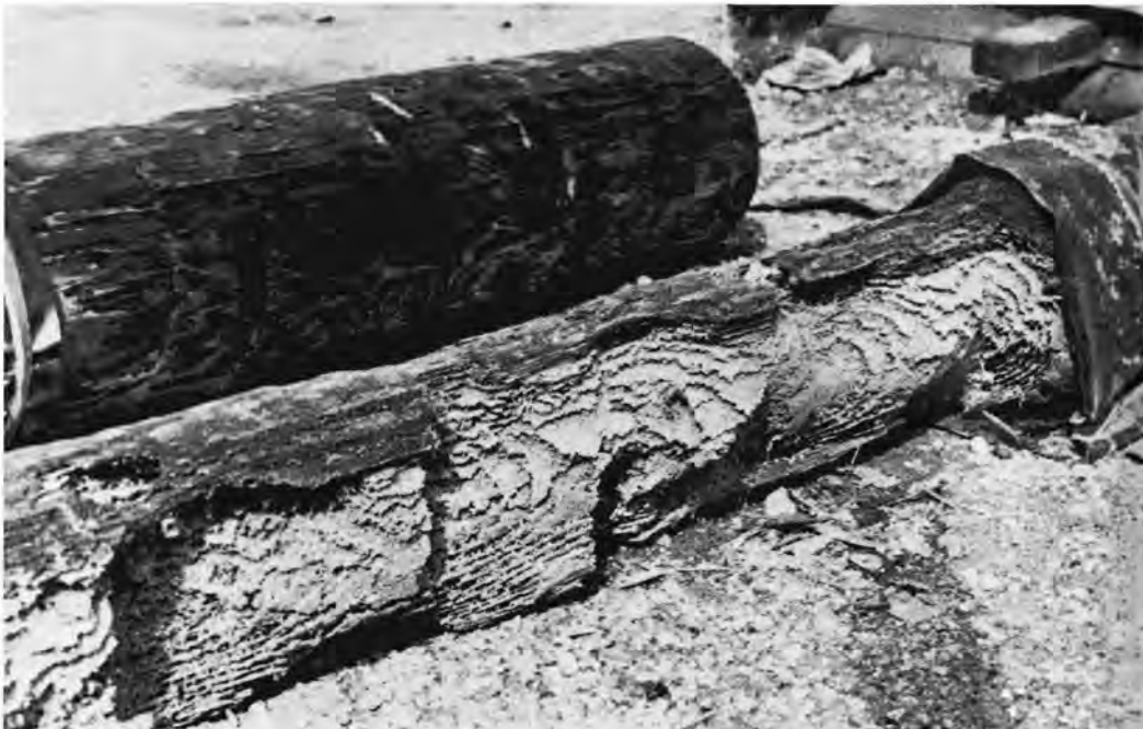
The pile in the foreground looked like the one above before Limnoria did their damage.
