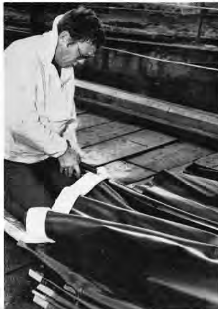
Impregnated polyurethane foam seal is being stapled across the end of Pile-Gard sheeting.
