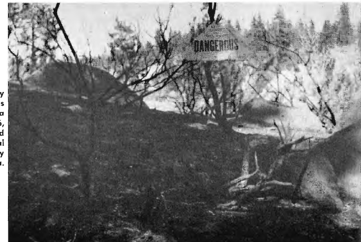
Fire destroyed many communication poles and trees in this area near Milepost 316, and blackened ground for several miles. Photos by Millers, Portola.
