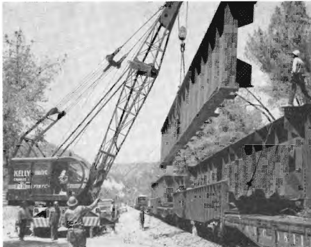
Beams from a steel fabricating plant in Chicago, weighing several tons, are unloaded at the site of a Western Pacific relocation bridge on the Feather River about a mile and a half east of Oroville. The bridge will be used when the rising water behind Oroville Dam inundates several miles of track. Oroville Mercury photo.
