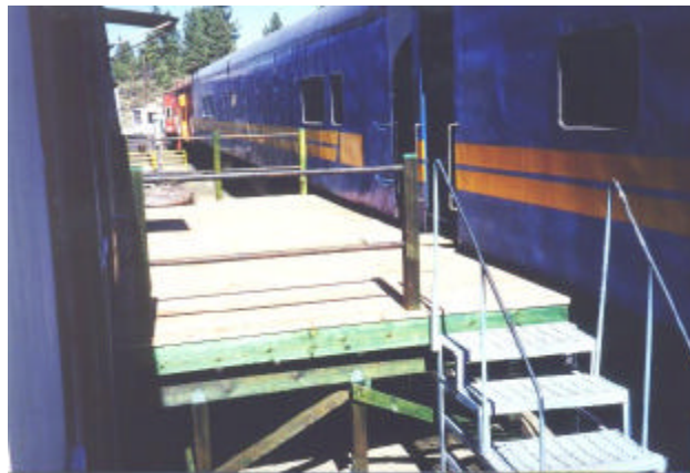
Now complete the new deck between the sleeper and shower car provides a walkway between the two cars as well as a place to bar-b-que lunch or dinner for our volunteers. - Norman Holmes
