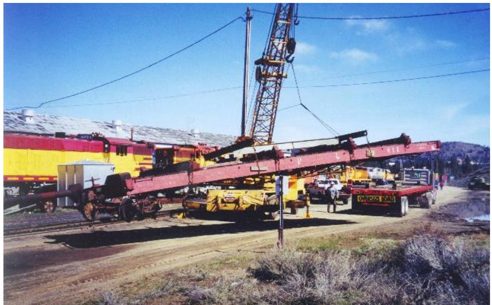
After being lifted from the truck trailer one of the flat cars is being swung around in preparation for setting it back on its arch-bar trucks. - Norm Holmes
