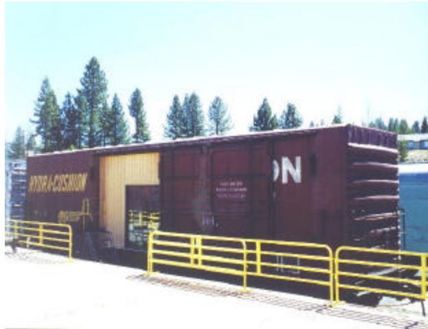
Our new library car is the culmination of many hours of work. Access to the interior of the car was made easier by framing in the opening of the plug door and installing a sliding glass door. This also protects the contents from the elements. - John Walker
