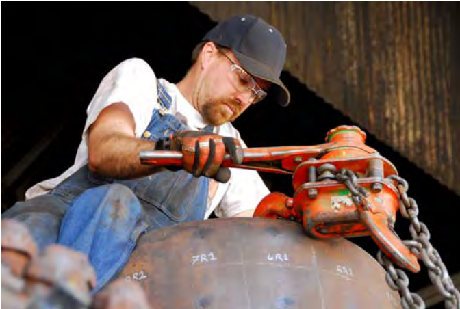
Erin Swain checks the rigging for lowering the power reverse from the side of the boiler.
