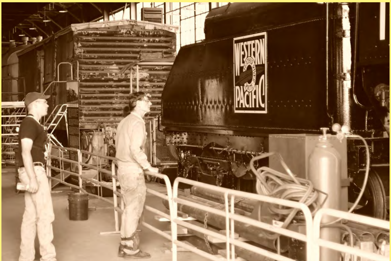
David "Fritz" Elems and Bob Sims discuss the finer points of reinstalling the wooden floor in the cab of the 165.
