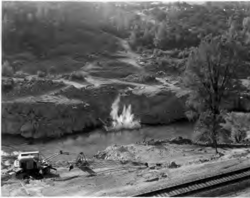
No. 168-1 9-19-58 Feather River Bridge. View of underwater blast at Pier No. 4 looking ahead on line at succeeding pier locations.
