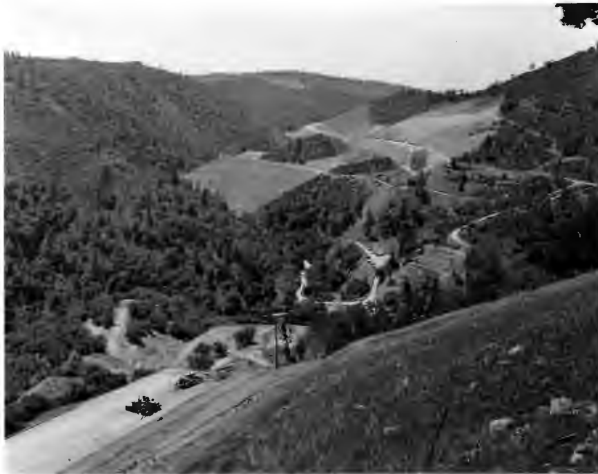
No. 690-8 5-10-60. West Branch Bridge. General view of bridge site, east abutment lower left at bulldozer - access road to intermediate piers, west abutment and piers near completion at top center.
