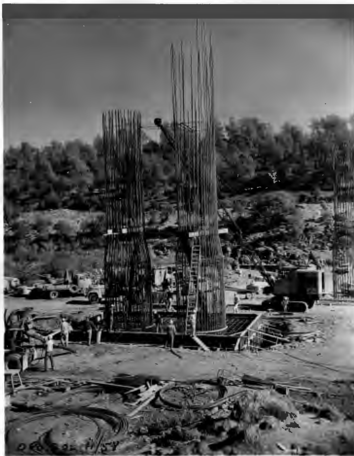
No. 202 11-7-58 Feather River Bridge. View showing men and equipment at work placing concrete on Pier No. 8.
