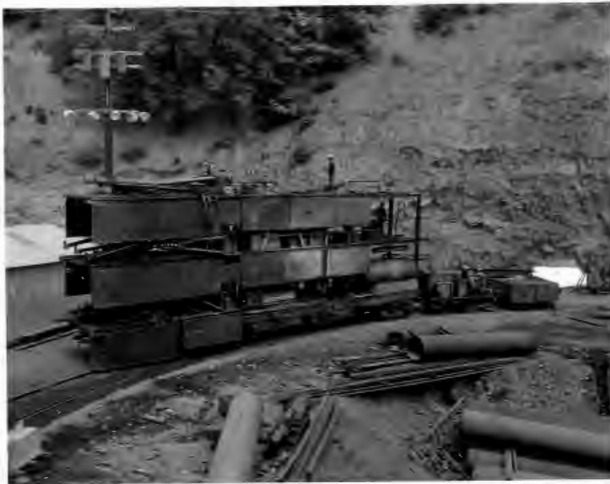
No. 149-9 7-29-58 Tunnels 4 and 5 (W.P.R.R. 7 and 8). View of drilling Jumbo being loaded with lagging prior to run into tunnel.
