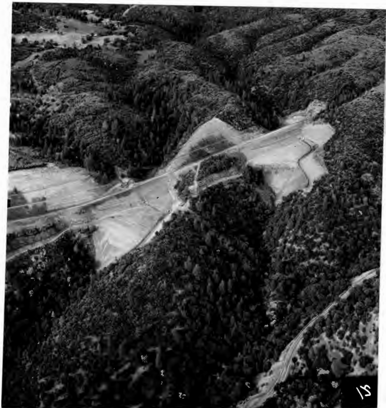
No. 853-12 11-28-60 Tunnels Nos. 2 and 3 (W.P.R.R. Tunnels Nos. 5 and 6). Aerial view of waste area right of Station 1065- and Station 1076 + . Grizzly Creek is passed through twin 126-inch culvert at right center.
