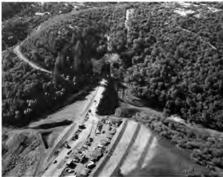
No. 562-4 1-15-60 Tunnels Nos. 2 and 3 (W.P.R.R. Nos. 5 and 6). Portal 2E interceptor ditch over Portal. Cut slopes and fill over 138-inch CIMP and 150-inch CIMP. Inlet to 138-inch CIMP at Station 1002+08.
