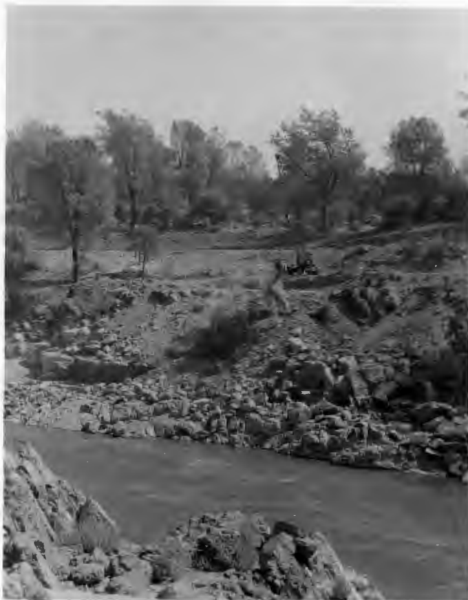
No. 157-3 9-8-58 Feather River Bridge excavation proceeding at Pier No. 2. Existing N.P.R.R. track in back- ground.
