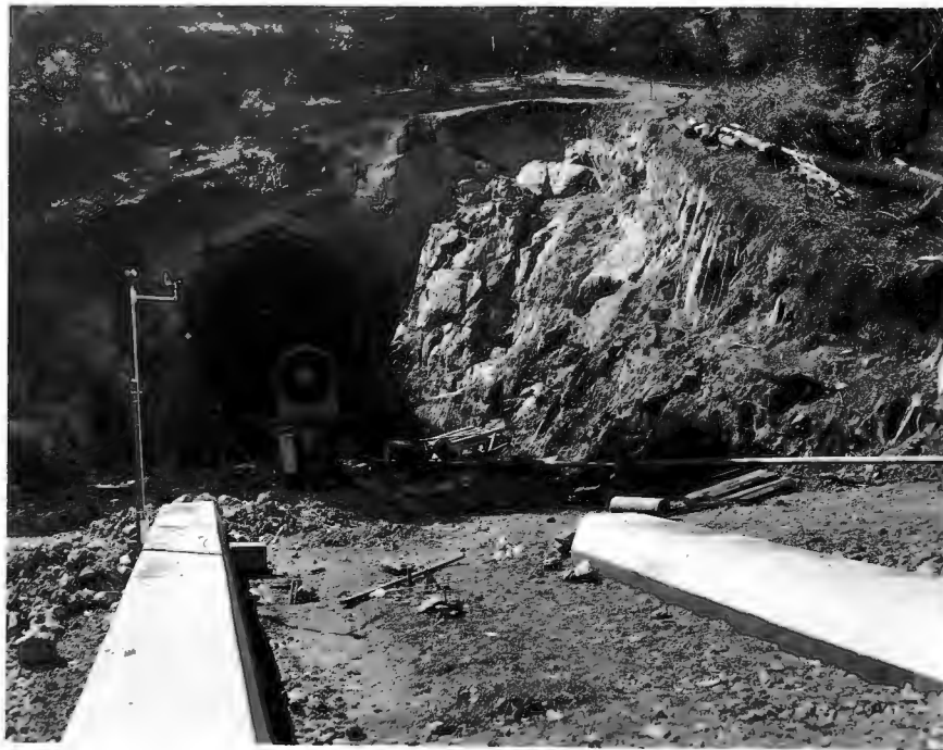
No. 490-1 9-21-59 Tunnels Nos. 4 and 5 (W.P.R.R. Nos. 7 and 8). East Portal Tunnel No. 5, Abutment No. 1, North Fork Bridge.
