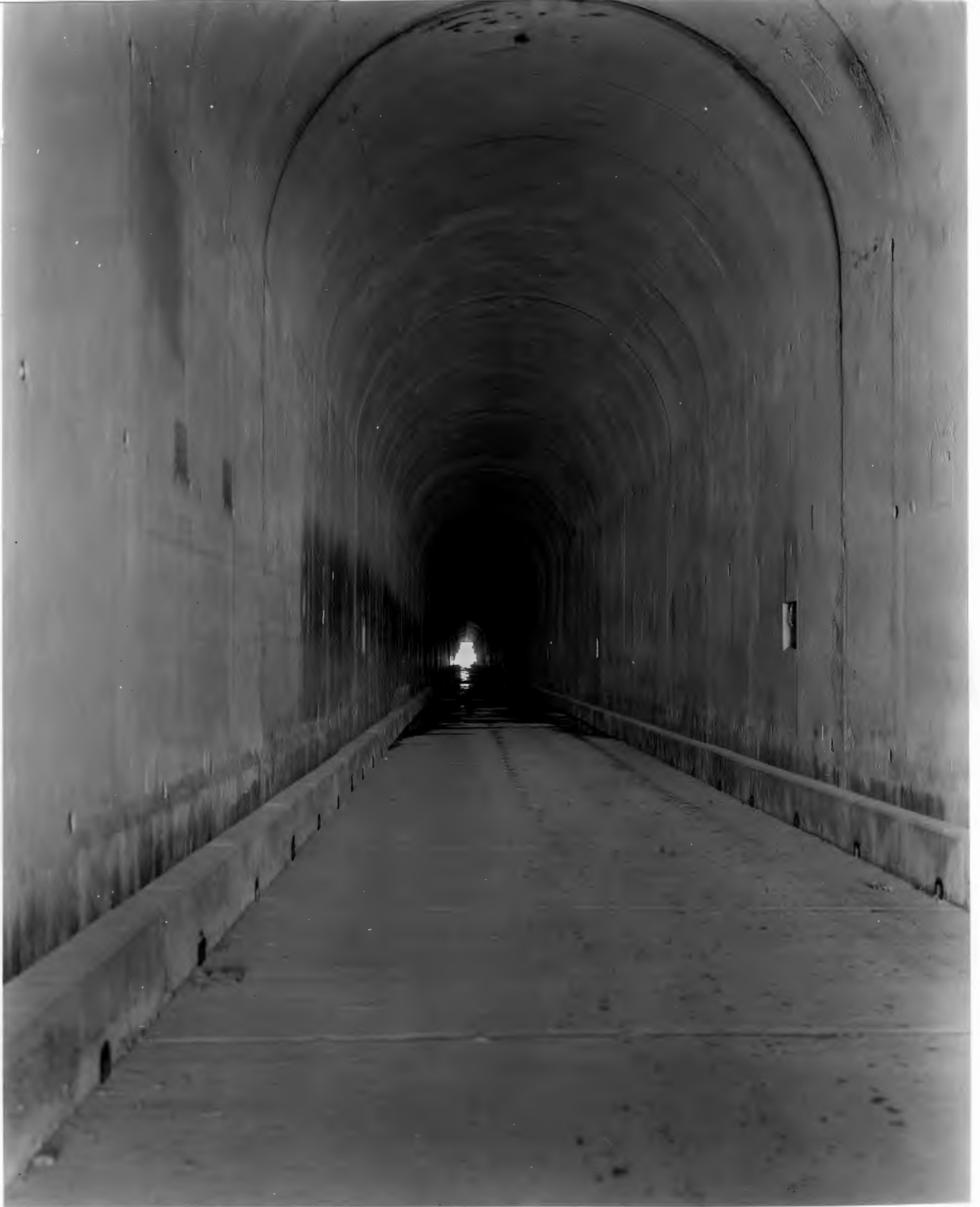
No. 857-1 12-5-60. Tunnels Nos. 4 and 5 (W.P.R.R. Nos. 7 and 8). Completed section of Tunnel No. 4. Portions of the invert are subject to standing water.
