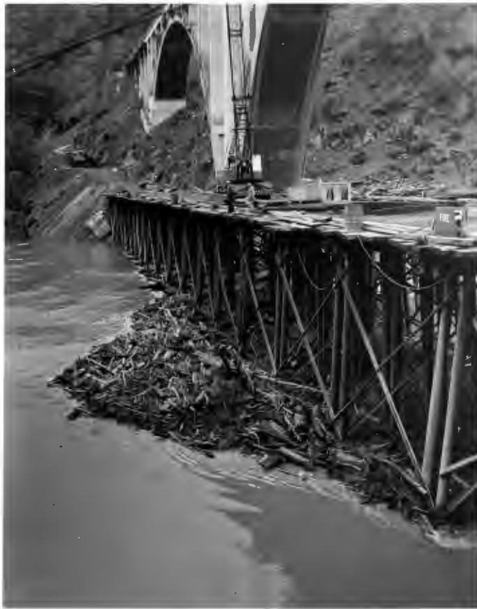
No. 582-1 2-9-60 North Fork Bridge. Debris piling up at the work trestle during high water.
