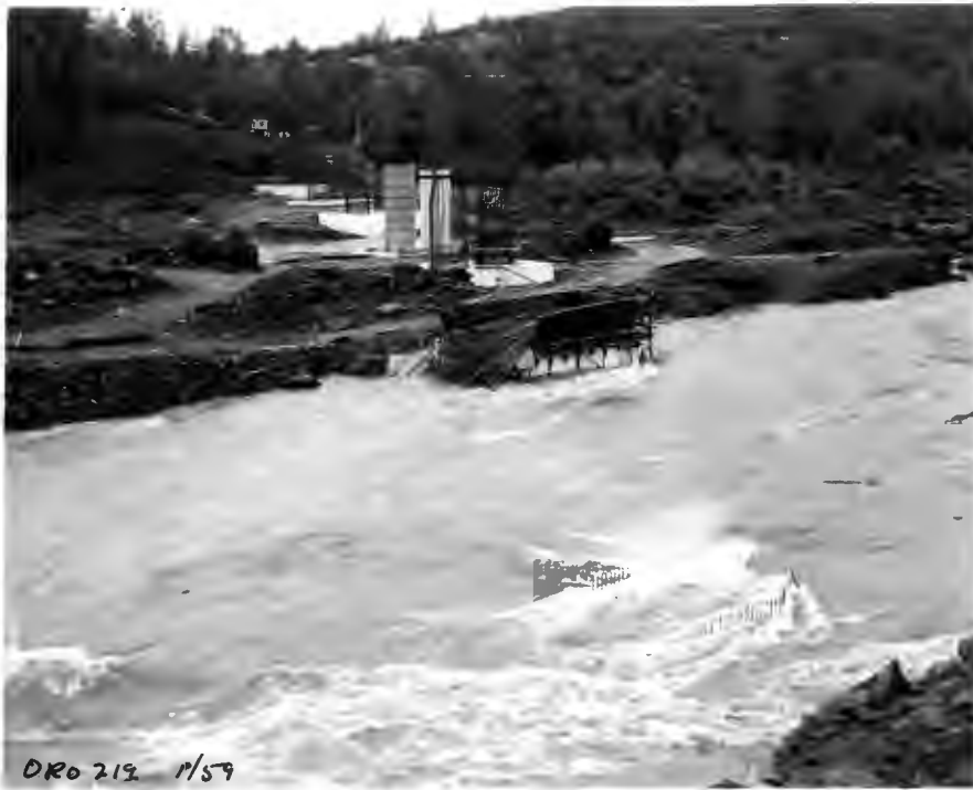
No. 219 1-12-59 Feather River Bridge. Looking ahead on line. Note reinforcing steel of Pier No. 3 in foreground. Collapsed reinforcing steel on Pier No. 4 across river.
