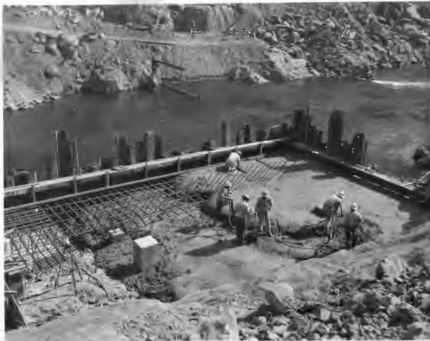
No. 189-3 10-16-58 Feather River Bridge. View back on line at concrete placing operation at Pier No. 4.
