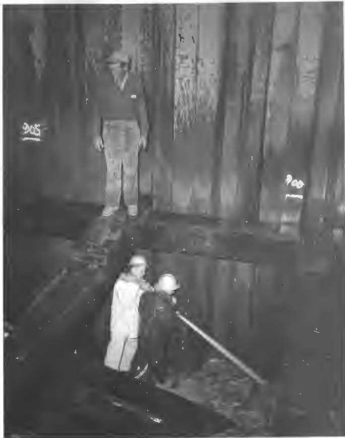
No. 191-1 10-16-58 North Fork Bridge. Washing down bedrock before placing reinforcing steel at Pier No. 3.
