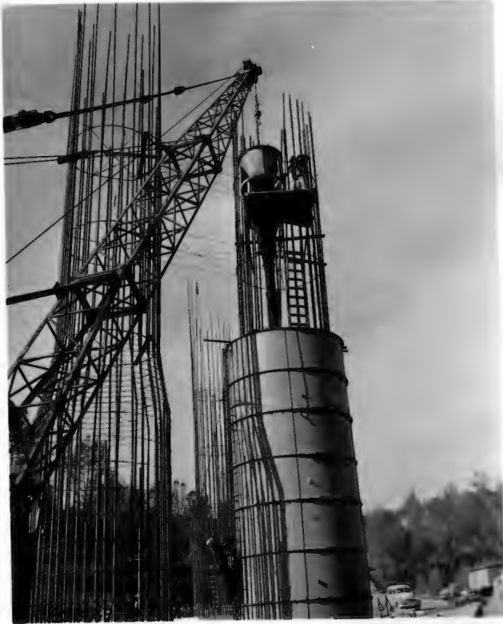
No. 227 12-19-58 Feather River Bridge. Close-up of concrete placing operation at Pier No. 6, using platform and tremie tube.
