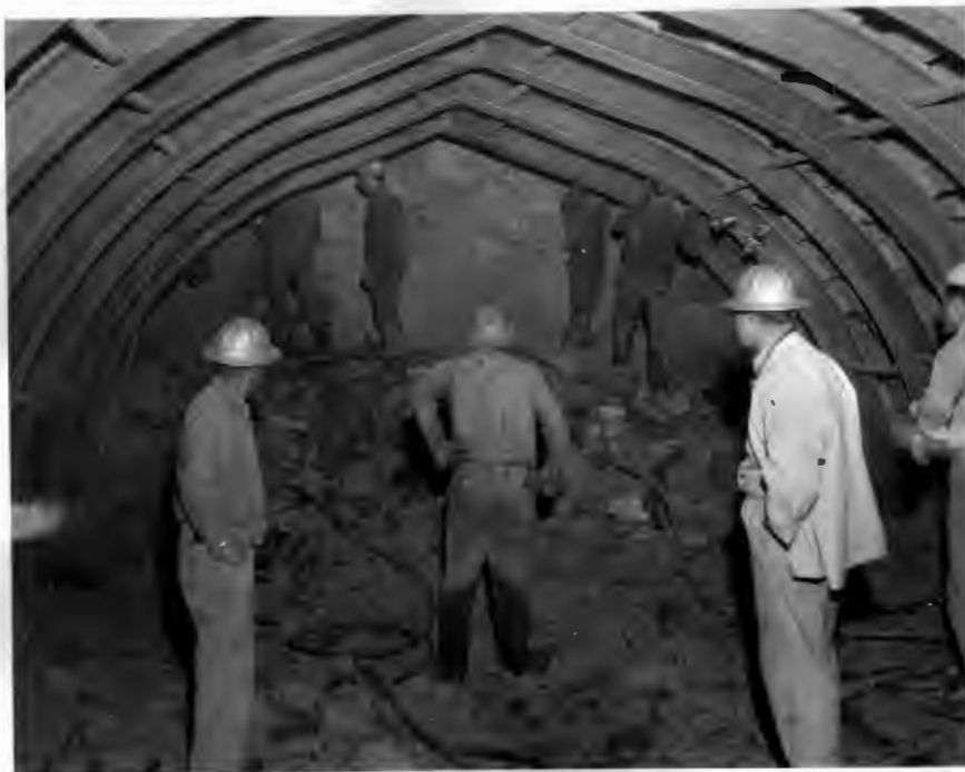
No. 188-5 10-25-58 Tunnel No. 4 (W.P.R.R. No. 7). Placing final lagging prior to holing out of Portal 4W.
