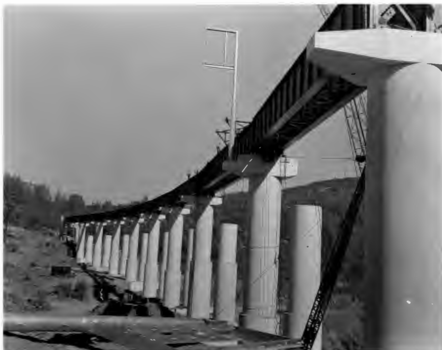
No. 426-7 7-27-59 Feather River Bridge. View of underside of in-place girders during erection.
