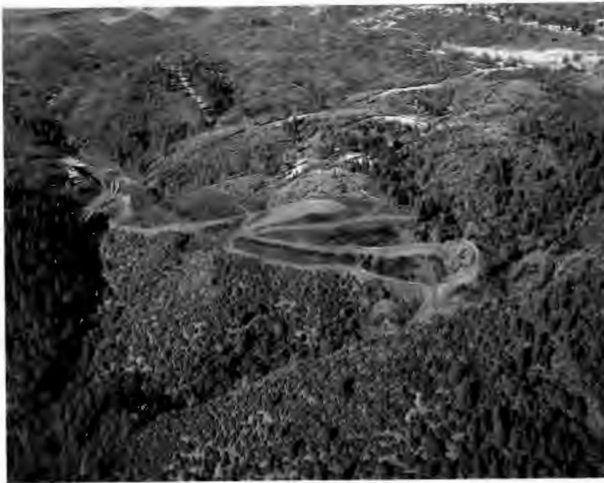
No. 561-1 1-15-60 Tunnels Nos. 2 and 3 (W.P.R.R. Nos. 5 and 6). Grading, clearing and excavation for Portal 3E.
