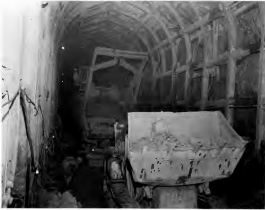
No. 154-1 8-18-58 Tunnels Nos. 4 and 5 (N.P.R.R. Nos. 7 and 8). Loading muck train after blasting. Note rock being moved to forward part of train.
