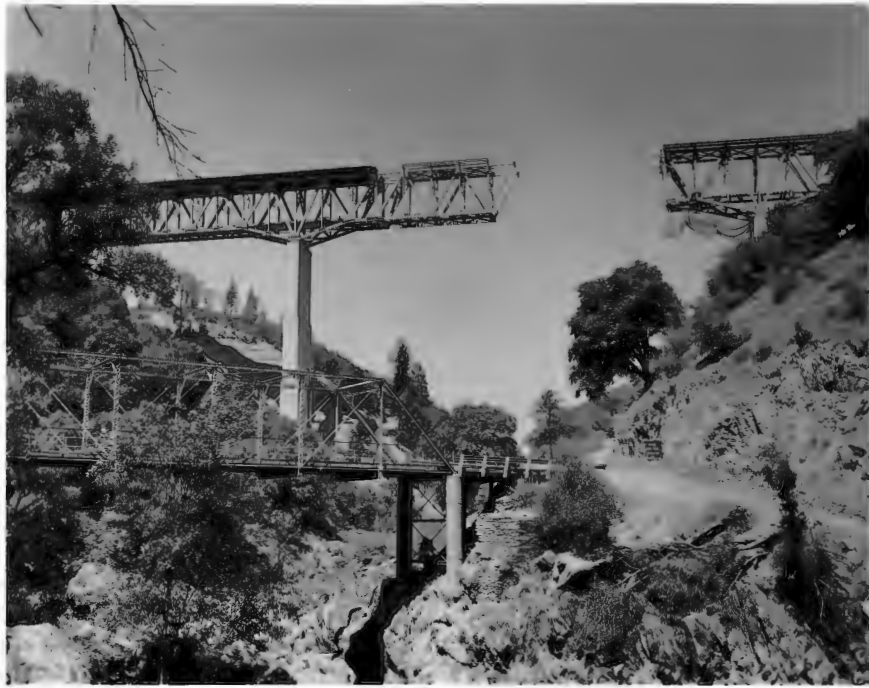
No. 1075-1 9-1-61 West Branch Bridge under construction. Old County Road Bridge in foreground.
