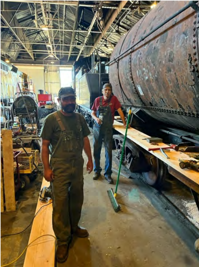
Channing Walker and Mike Waters putting the running boards on the Steam Department fuel tank car - 6/30/22.
