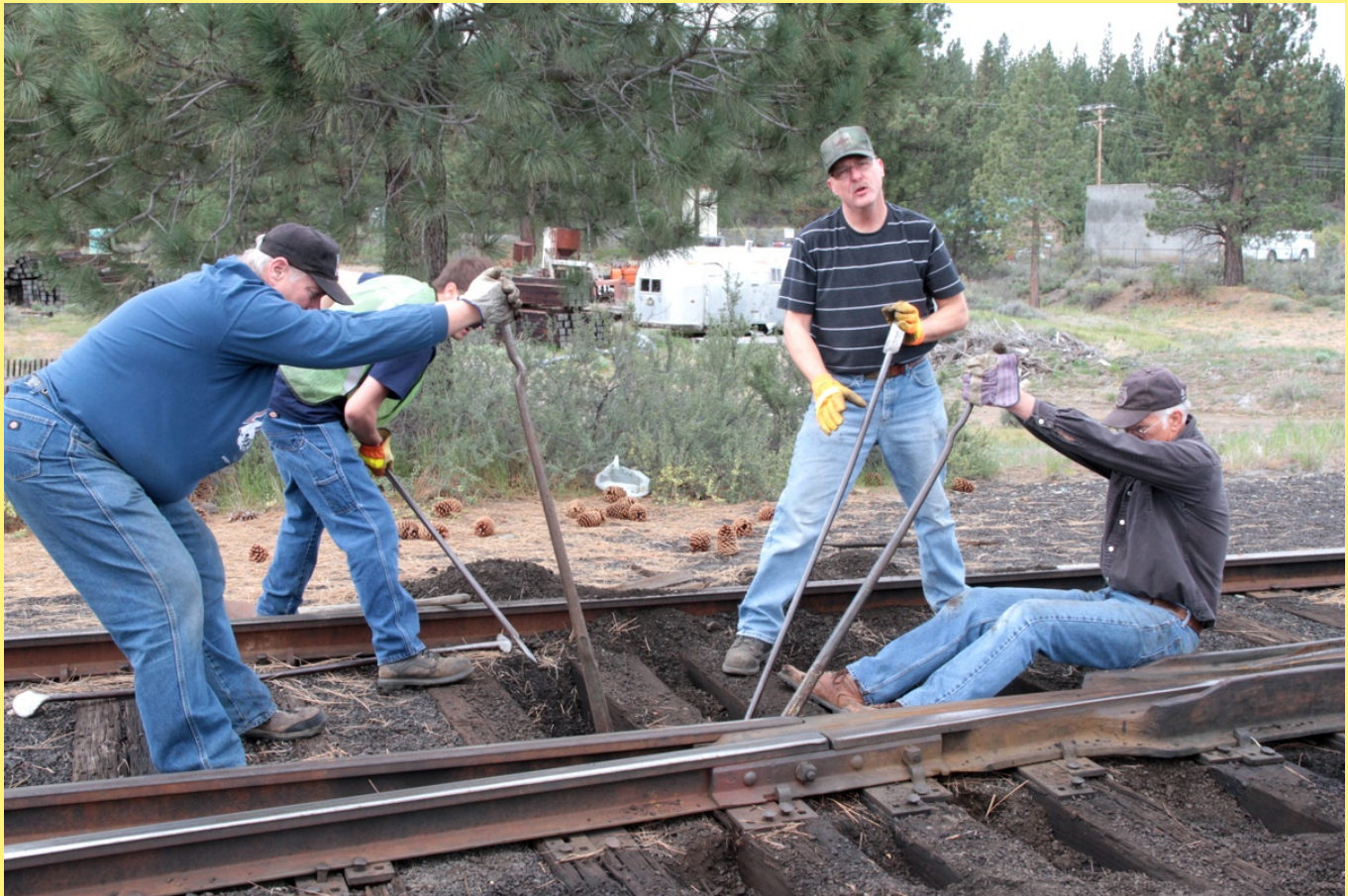
Greg Elems explains the efforts of volunteers doing track work to the photographer on 10 May, 2014. The ties under the switch frog are being raised and tamped to correct settling that has occurred over time. Pictured left to right: Rick Gruninger, Matt Elems, Greg Elems, Duane Vander Veen.
