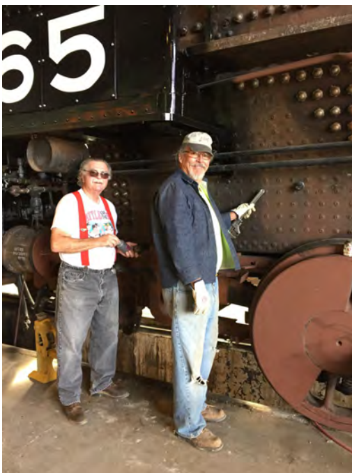
Hank Stiles and Mike Mehcam installing washout plugs. - photo by Dick Couden
